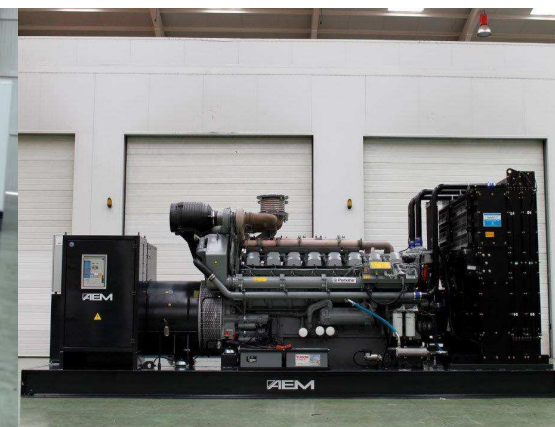
1500 KVA's POWER PLANT (3 x Deutz 500 KVA's) TAILOR CONTROL PANEL 3 Synch Gensets in mode stand by of the the national grid
